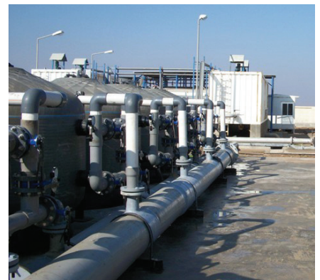
▲ Each plant consisted of 10 x Micron SMD2000 Filters.
