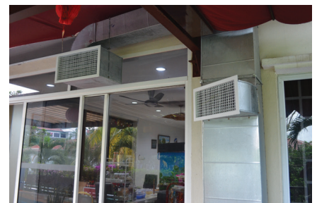
The Ducting System for Channelling Cooled Air Back into the House
