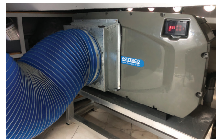
Duct Connected to the Heat Pump Unit
