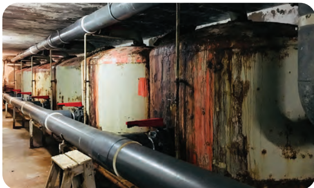
Corroded metal fabricated filters
